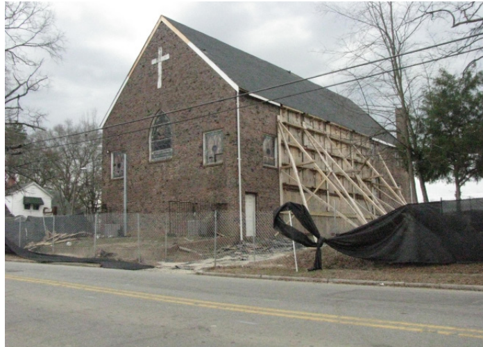
The building, on the corner of Main Street and South Holman Street, is undergoing work on imminent structural concerns. (Photo by Catherine O'Neill)
